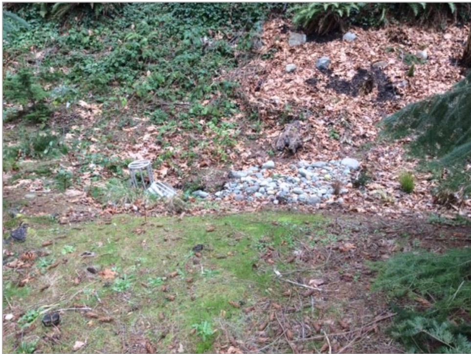
Photo 8 — New catch basin and stormwater pipe at 8100 SE 48 th Street, which contributes runoff into subject stormwater pipe. Catch basin drains directly downhill through 8101 SE 48 th Street to subject .
