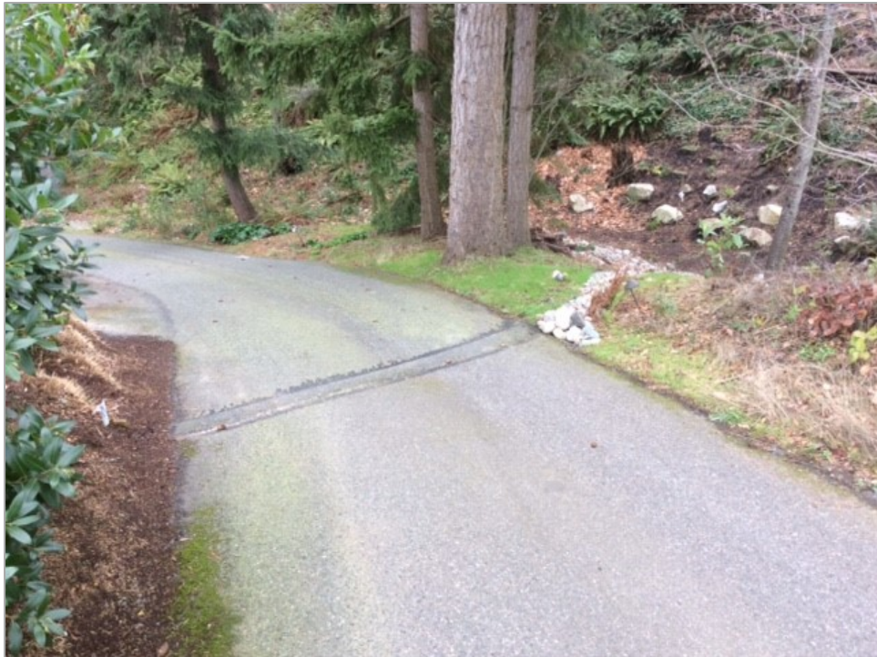
Photo 6 — New runoff collection on private shared drive to 8101 and 8105 SE 48 th Street, which contributes runoff into subject stormwater pipe, which appears relatively recent.
