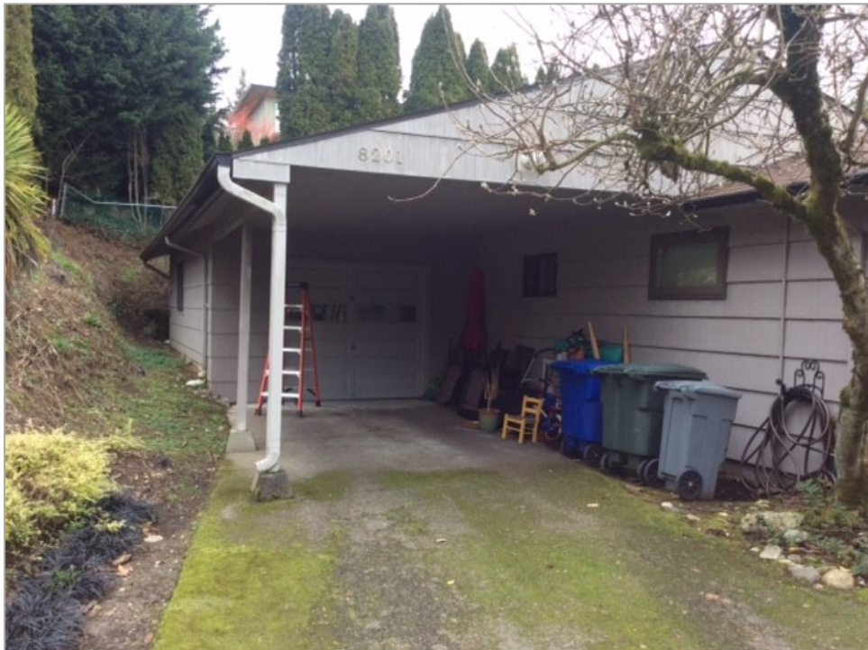
Photo 4 — Driveway and roof drains at 8201 SE 48 th Street, which contribute runoff into subject stormwater pipe.
