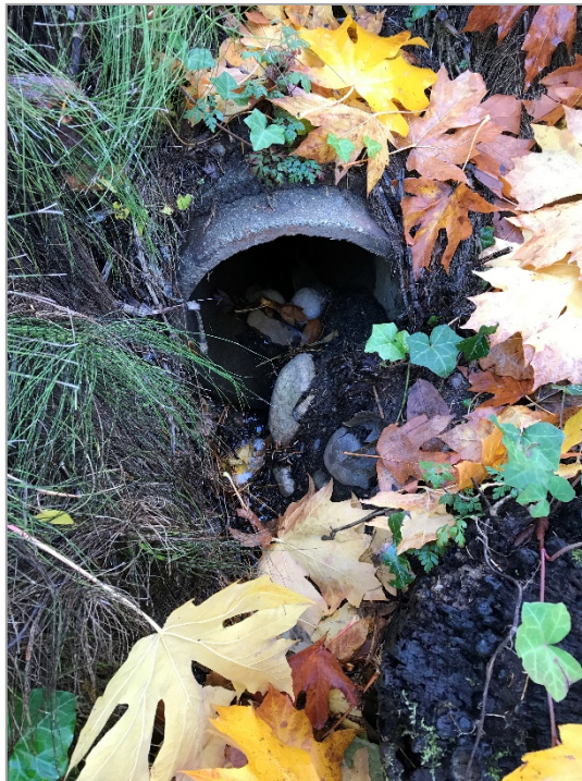
Photo 4 — SE 48 th Street stormwater pipe outlet.
