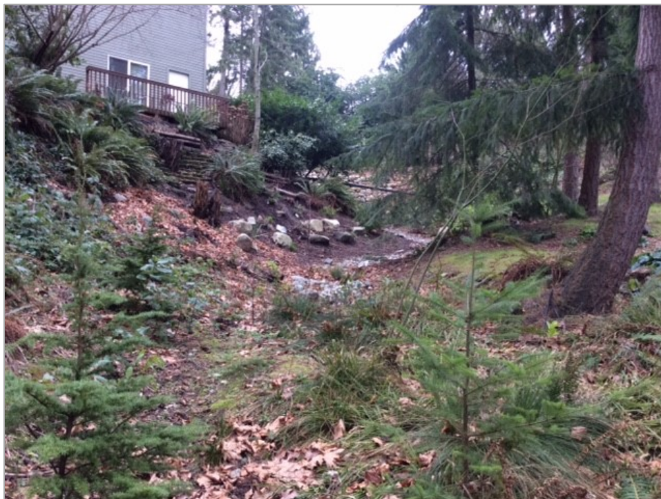
Photo 9a — View of new catch basin and stormwater pipe from downslope. Several trees were removed during installation of drain, causing an increase in runoff as well.
